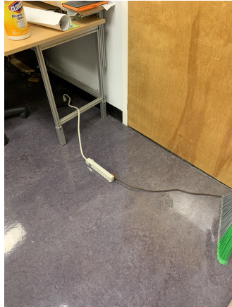
Refrigerator into power strip.
