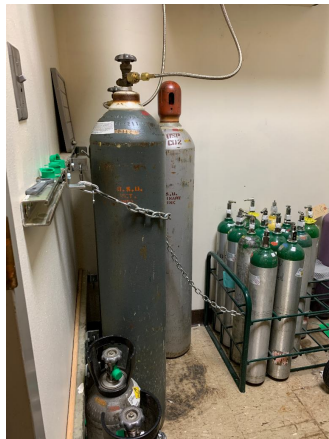
Gas Cylinder Room
