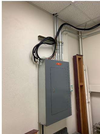
Room 428 Exposed Wires
