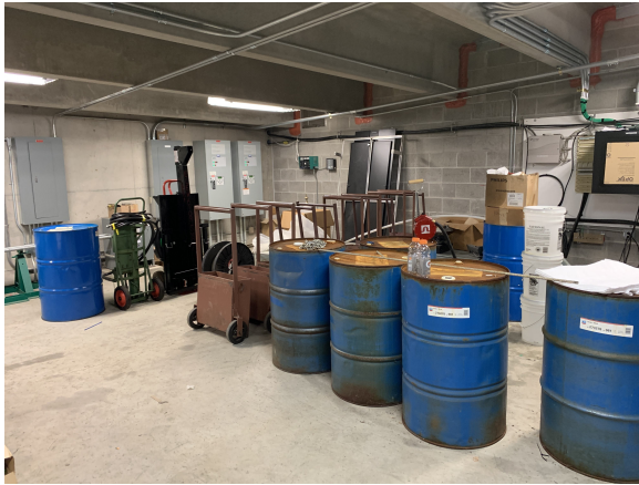
First Floor Electrical Room
