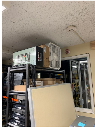
PEAK Storage Room
