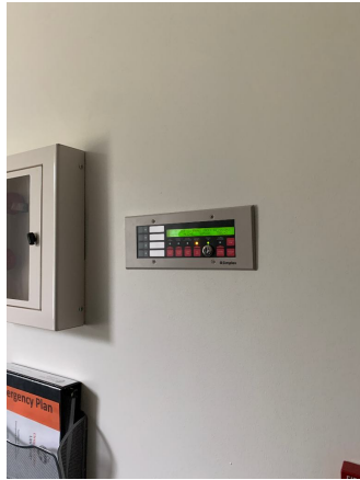
Fire Alarm Panel
