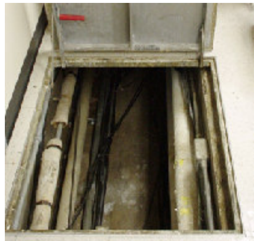
Live steam lines? Electrical lines?
