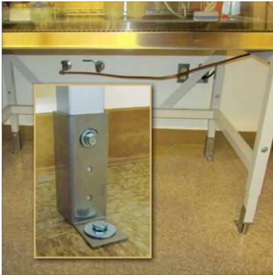
Biological safety cabinet anchored to the floor with a metal bracket
